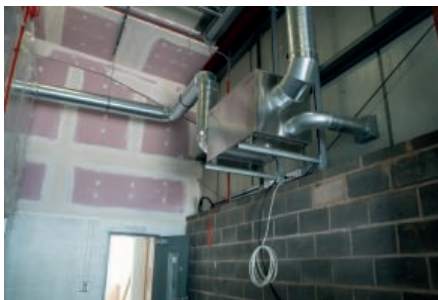
The storage pod is designed to keep itself cool with this dehumidifier to assist when required.
